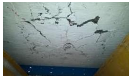
Fig. 14. Crack Pattern on Top of Slab
